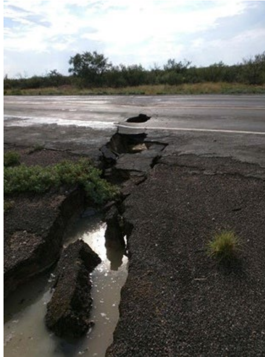
Figure 6. FM 1053 Sinkhole in Pecos County, Texas 78
