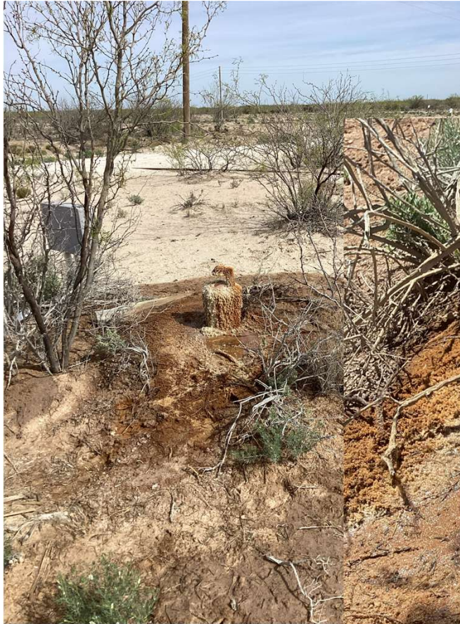
Cathodic Protection well
